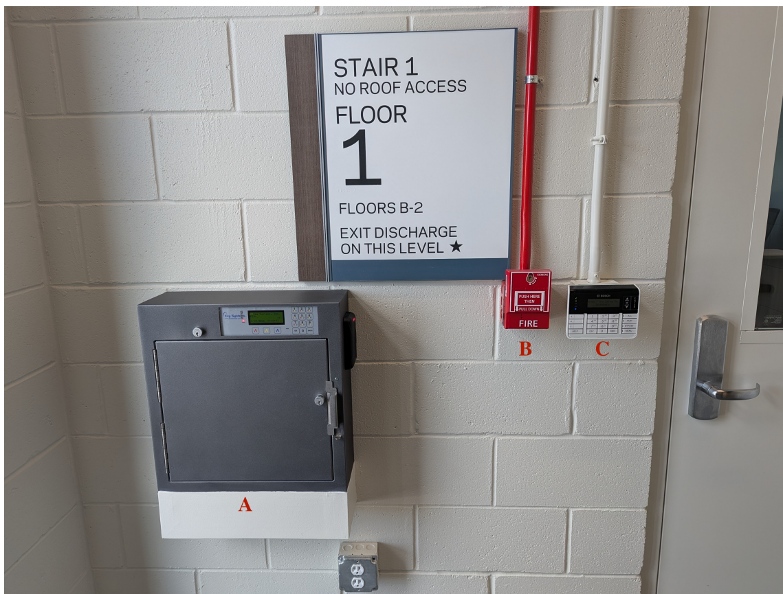
Figure 9: Reception of north staff entrance, containing: (A) lockbox, (B) fire pull, and (C) security keypad.
