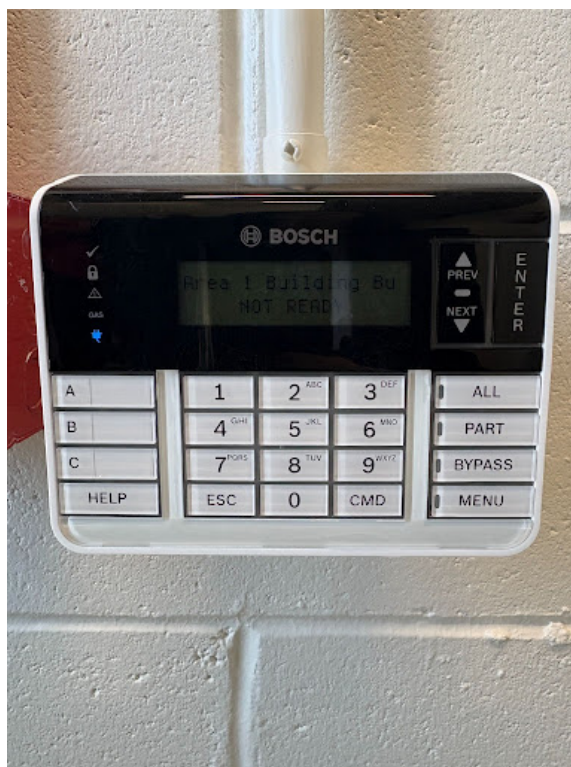
Figure 8: VFPC alarm system at staff entrances.
