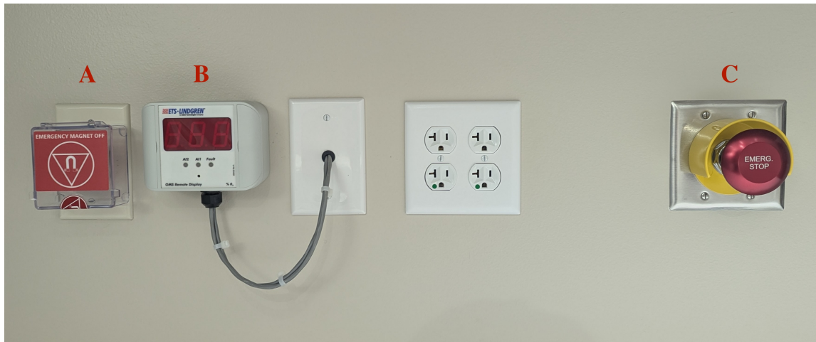
Figure 3: Magnet Room button wall. A Quench. B Oxygen sensor, alarm. C Emergency Power Off.
