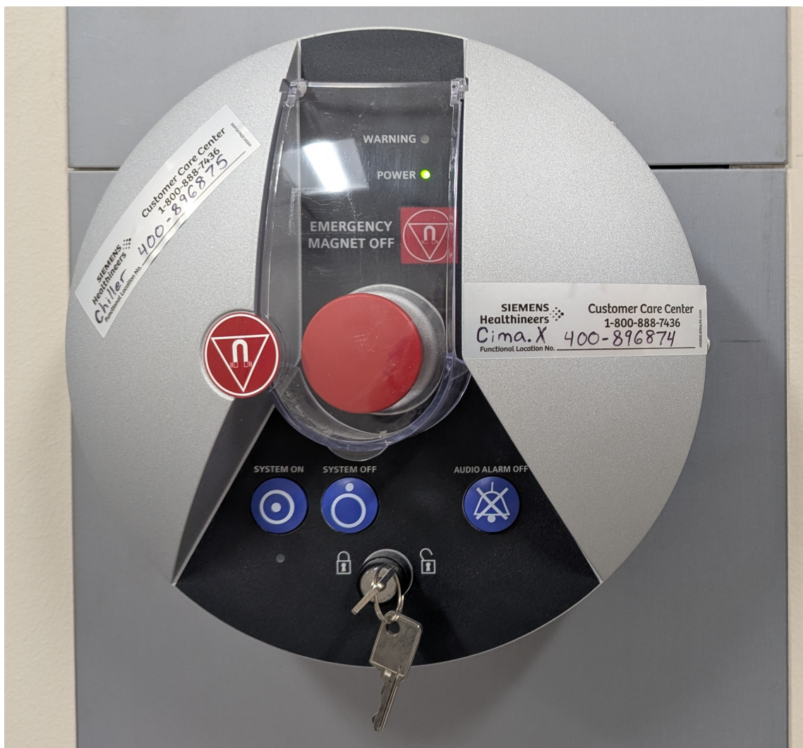
Figure 2: Control Room MRI quench button.
