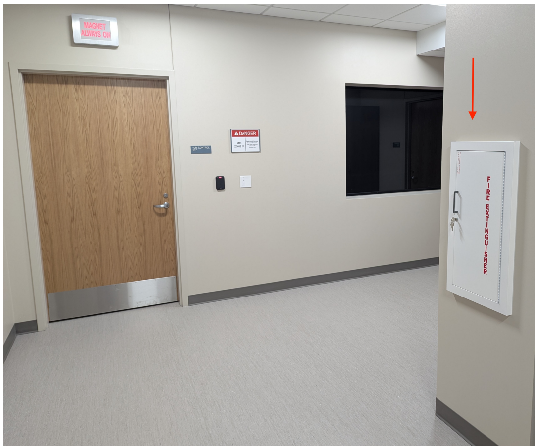
Figure 3: Zone 3 (B15) fire extinguisher location (red arrow).
