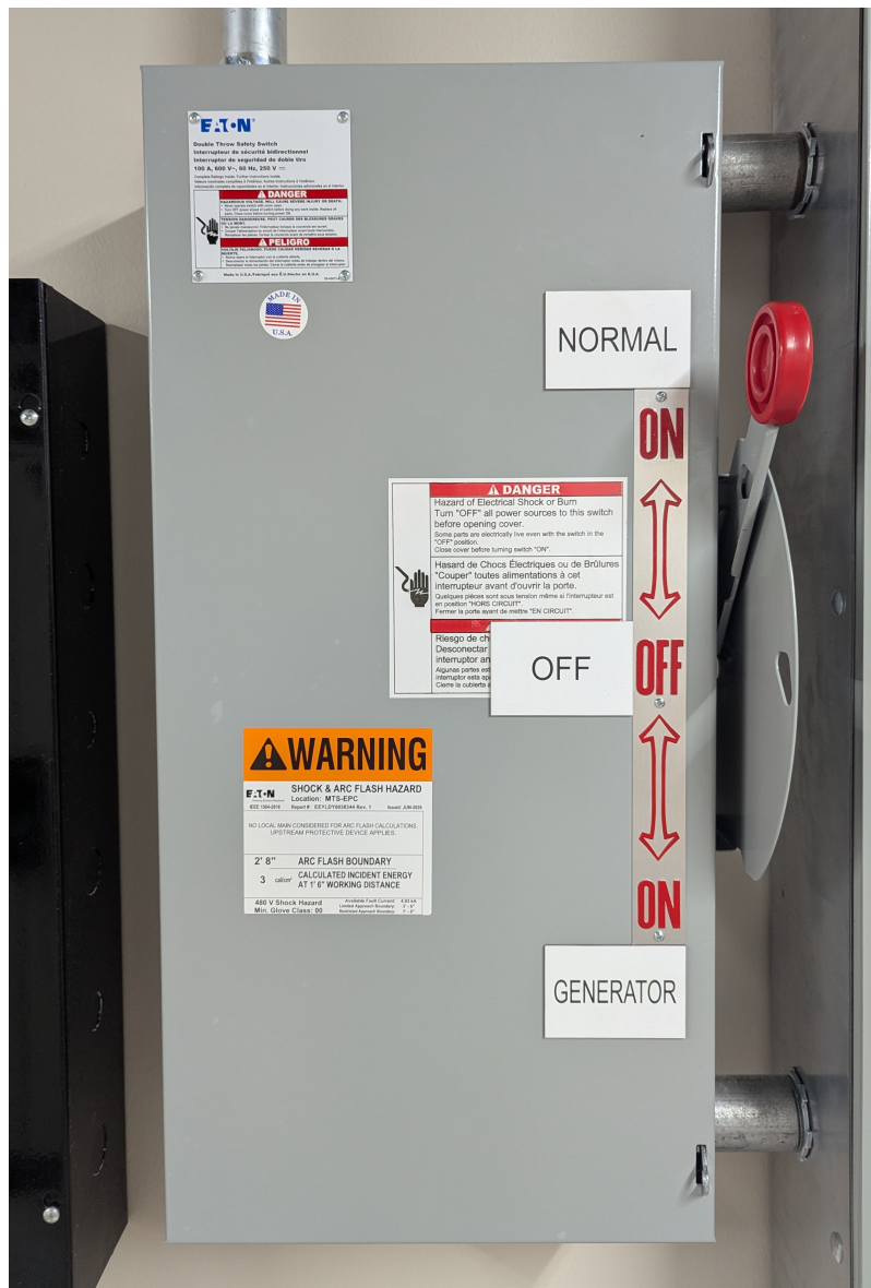
Figure 9: Cooling pump power switch.
