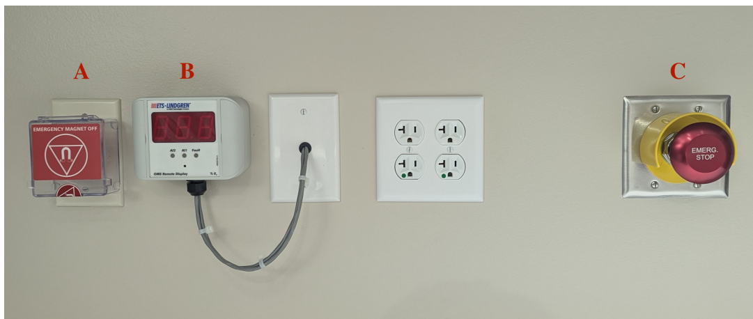
Figure 1: Magnet Room button wall. A Quench. B Oxygen sensor, alarm. C Emergency Power Off.
