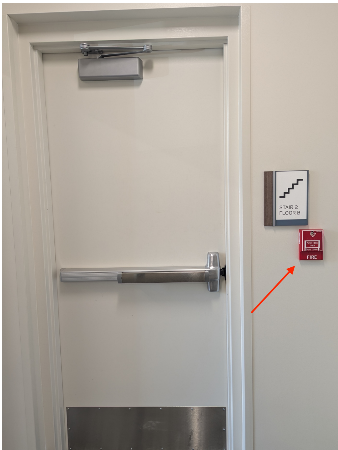
Figure 5: Lower level fire alarm, south door (red arrow).
