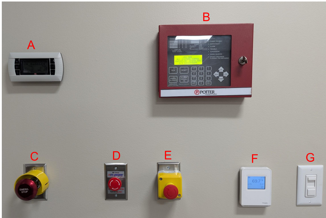
Figure 2: Control Room button wall. A Haskris Coolant Sounder. B Fire System Board. C Emergency Power Off. D Magnet Door release. E Unknown (potentially electric power off). F Thermostat. G Light switch.
